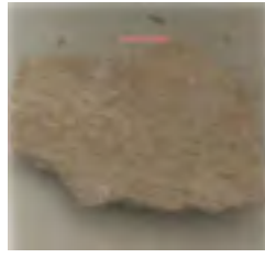
Part of the mortar from the exterior walls
